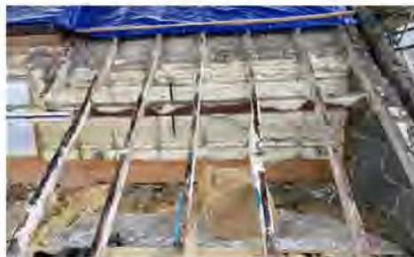
A surveyor's case of a roof damaged by spray-foam insulation
